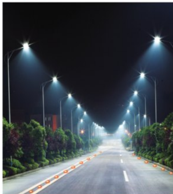
Street light and Reflector
