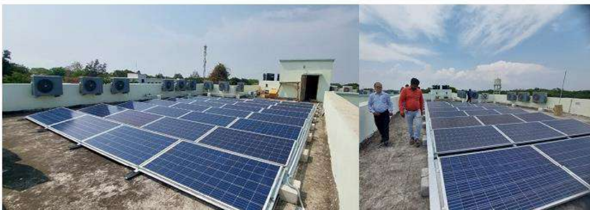
30 Kwp Roof Top Solar Plant (RTSP) installed successfully on the roof of Central Instrumentation centre, BU 120 Unit of Electricity per Day
